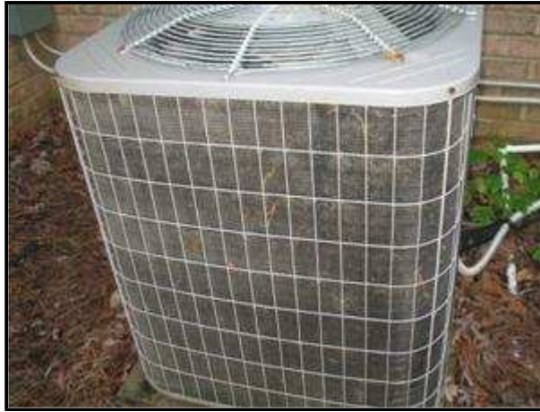
8.8 Picture 1 dirty coils
