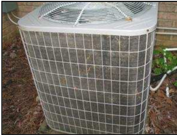
Item 16 - Picture 1 dirty coils
