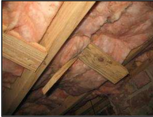
5.3 Picture 1 Bridging not nailed
