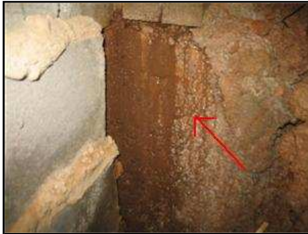
5.0 Picture 2 water intrusion
